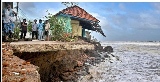
Swept away: A home destroyed by the cyclonic swell in Kakinada district of Andhra Pradesh on Tuesday. K.R. DEEPA
