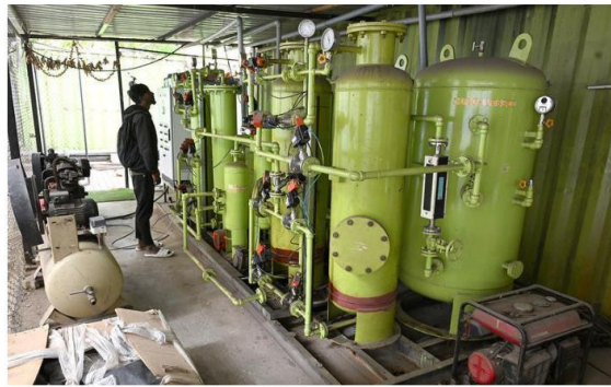
A biogas plant at the Waste-to-Energy unit in Koramangala in Bengaluru. J. ALLEN EGENUSE
